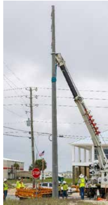
Crews install a concrete power pole in Northwest Florida to improve resiliency during hurricanes and severe weather and also enhance reliability year-round.
